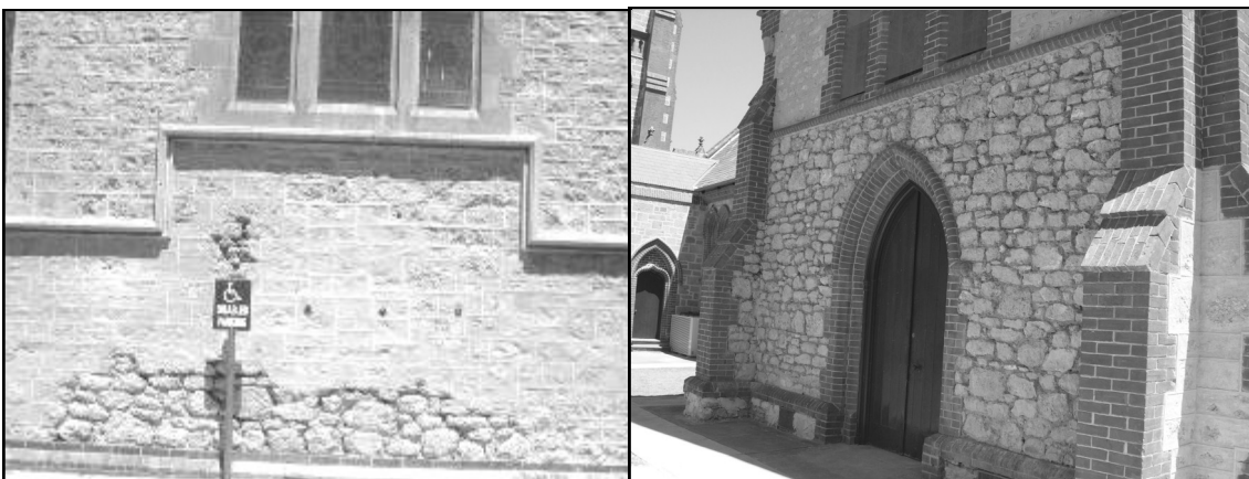
Examples of restoring the walls that have had the damaging cement mortar removed, and are now ready for the limestone mortar.
